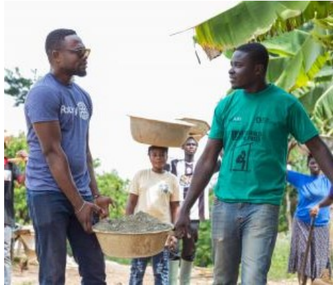
Cosmos Segbefia, a member of the Rotary Club of Sekondi-Takoradi, and Derrick Ababio Kwarteng, of Global Communities, assist with the construction of a borehole in the Western Region of Ghana in 2018. A report by Johns Hopkins University prepared for Rotary International estimated that Rotary members provide about 47 million hours of volunteer effort a year at an estimated value of $850 million.
